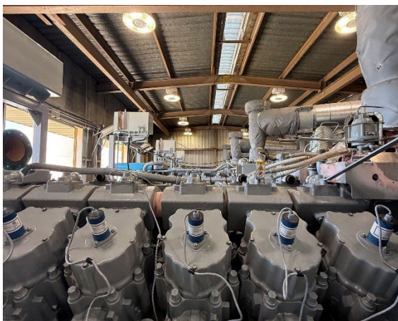
Removed Coolant Manifold at PP3
