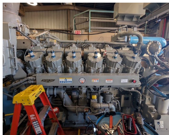
New Coolant Manifold at PP3
