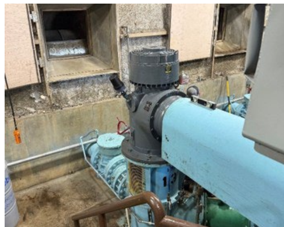
Installed PP1-E3 Gearhead
