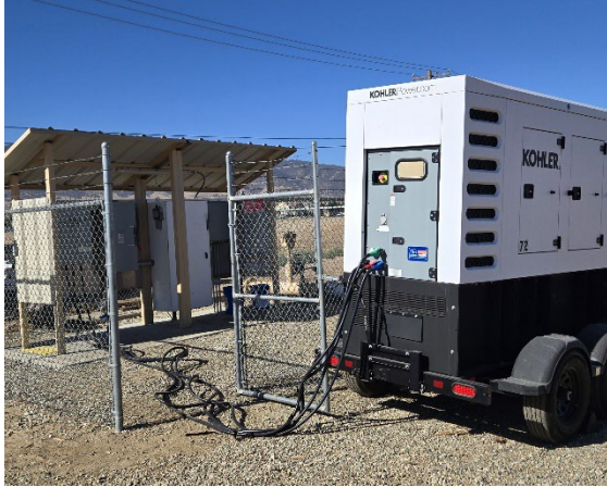
Running Nunes Well from Generator
