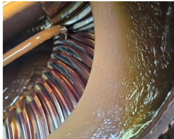
Damaged Gear Sets on PP1-E4 RA Drive
