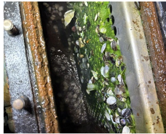
PP1 Heat Exchanger Screen
