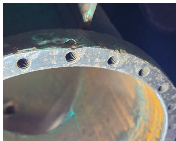
Worn Discharge Head/Column at PP4-E2
