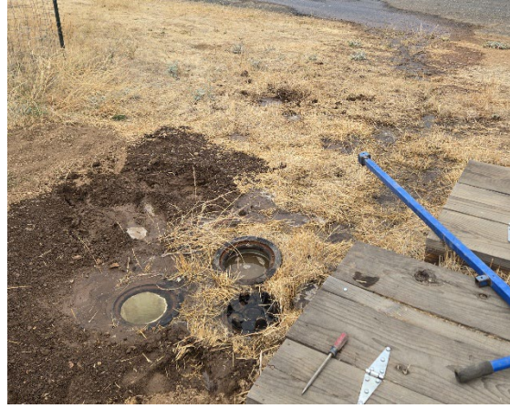
Leak on Neely Ave.
